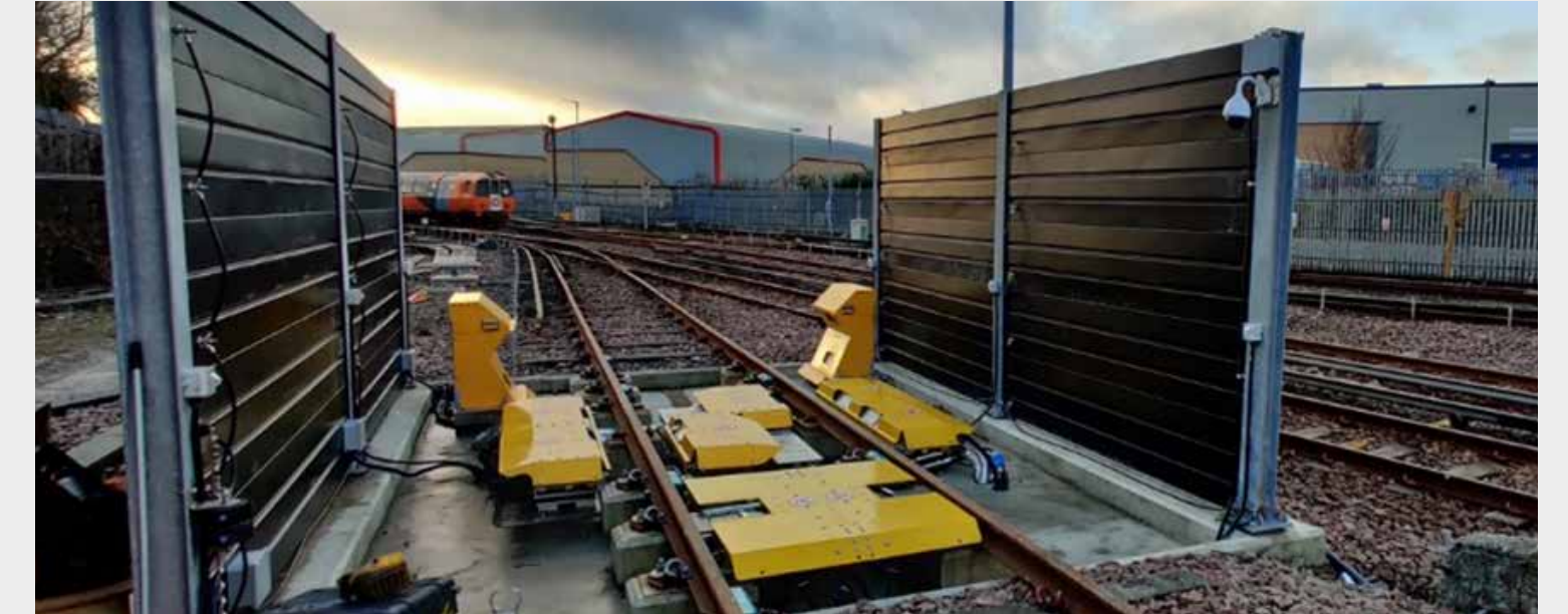
Automatic Train Inspection (ATI) accepted and operational.
